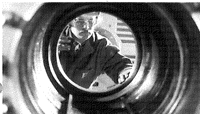
Step 15 Before installing the spare cartridge, the sealing surfaces inside the pump casing are inspected to make sure they are in good shape.
