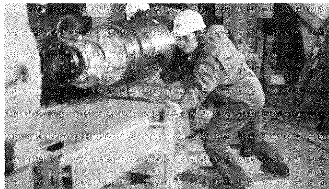
Step 16 Installing the replacement cartridge in the casing shell involves the same basic procedure in reverse. Once again the carriage is rolled up to the pump and bolted on. This time the cartridge is already in place on the carriage.
